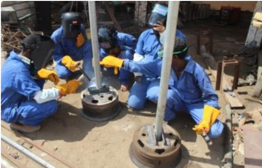
Brothers Welding Group working on poles for internet installation for a local school
